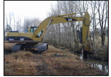
The District's Cat 325 excavator was used to dig out a local tax ditch.
